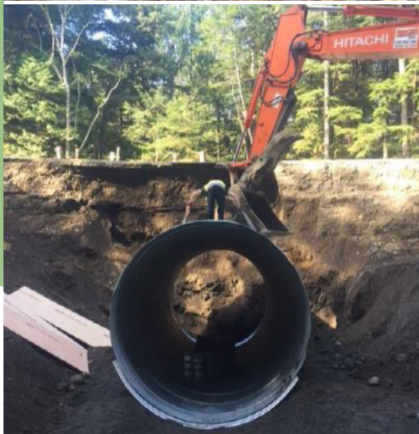
(Top) Inlet of concrete culvert in Muthmumc Creek (Creek 1) prior to replacement
